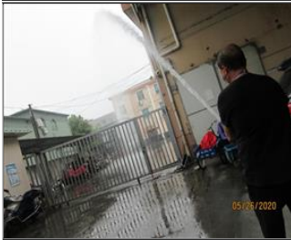
External photo(s) of the production unit(s) Fire hydrant testing onsite.jpg
