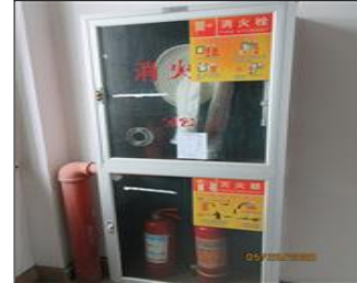
External photo(s) of the production unit(s) Fire hydrant and fire extinguisher.jpg
