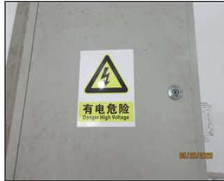
External photo(s) of the production unit(s) Electric box with warning sign.jpg
