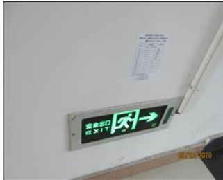
External photo(s) of the production unit(s) Evacuation direction sign.jpg
