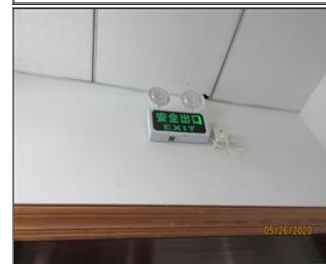
External photo(s) of the production unit(s) Safety exit sign and emergency light.jpg
