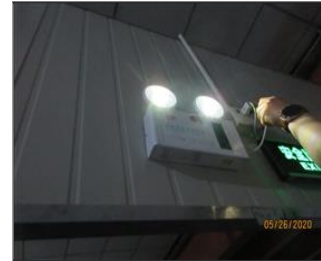
External photo(s) of the production unit(s) Emergency light testing onsite.jpg
